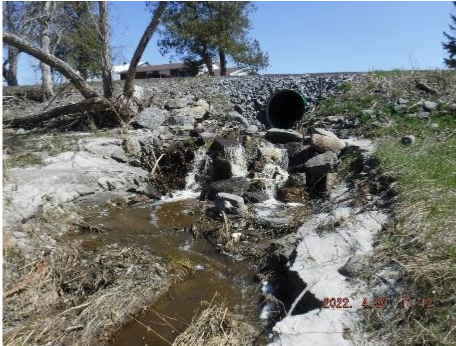
Photo 16: Drop of 1.5 m below the culvert under Pitch Off Road (April 29, 2022)
