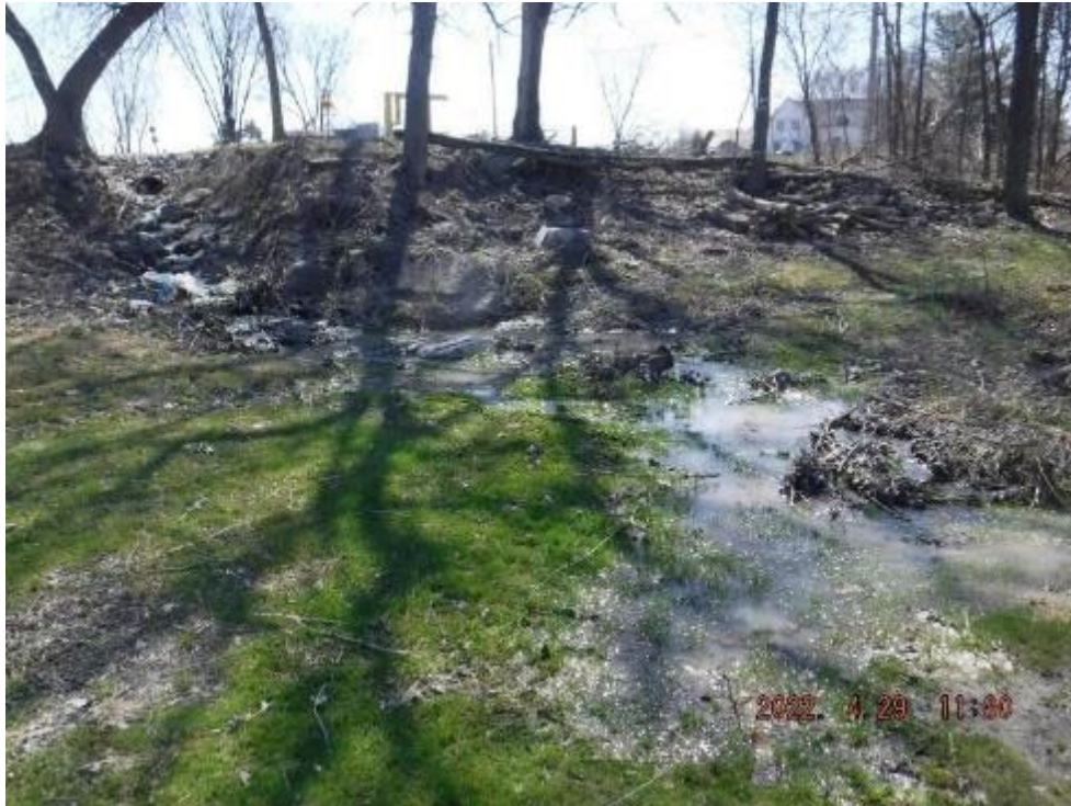
Photo 9: Looking upstream from the South Nation River at the culvert under Pitch Off Road Concession Road 5 north ditch and the lack of defined channel (April 29, 2022)
