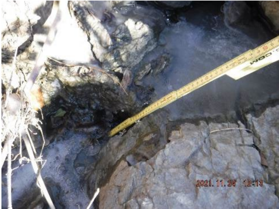
Photo 11: Looking at the step (fish barrier) in the north road ditch of Concession Road 5 (November 24, 2021)
