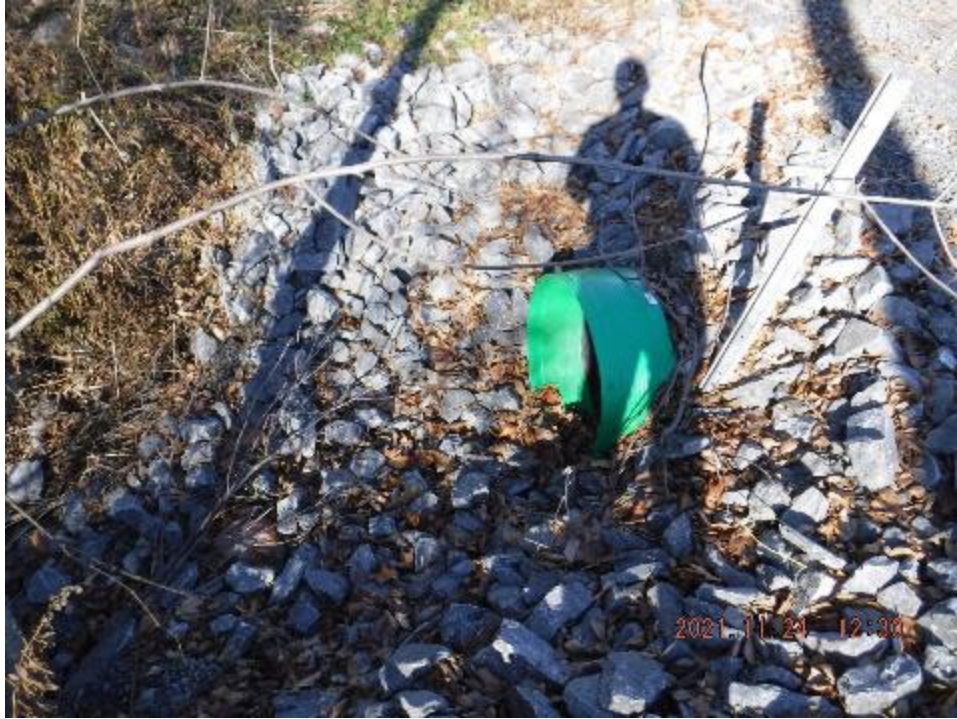
Photo 4: Culvert under Pitch Off Road for the flow coming from the south ditch (November 24, 2021)
