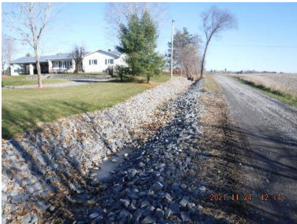
Photo 10: Looking upstream at the north road ditch along Concession Road 5 at the area that flow passes through rip rap (November 24, 2021)
